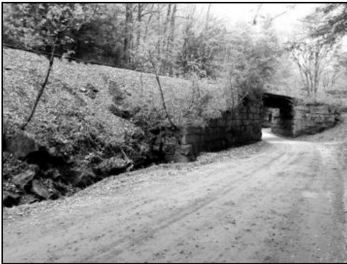
Cavendish Gulf Road underpass heading south. The rubble embankment to the left is scheduled to be replaced with a block retaining wall during the summer of 2015 by the Vermont Agency of Transportation.
